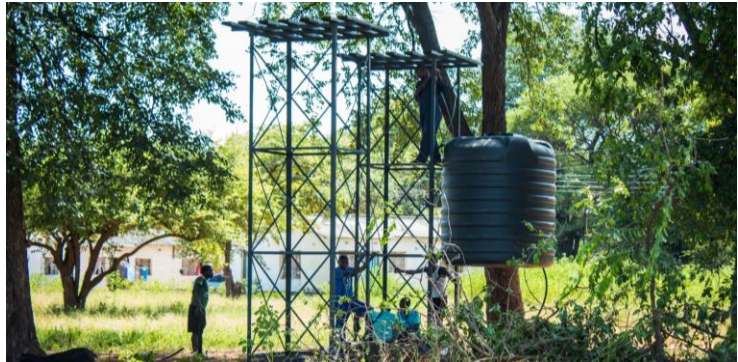
Water stands for 2x 5,000l tanks at each school: constructed and tanks hoisted on top of stands to gravity feed reticulation pipes; Local authorities are still to conduct a final inspection before the system can be “handed-over” to the schools.
