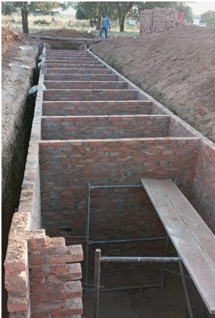
New toilet block (for students) under construction: foundations and septic pit (3m deep) for 14 toilets; both toilet blocks (students and staff) are expected to be completed during July/August 2022.
