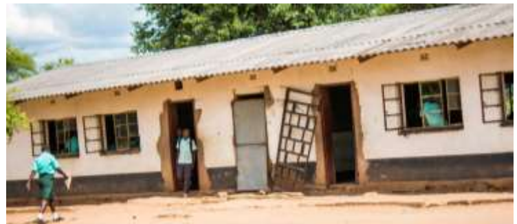
Hwata Secondary – March 2022, before repairs
