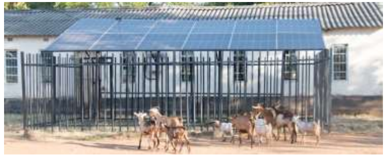
Solar panels mounted and fenced to protect from livestock
