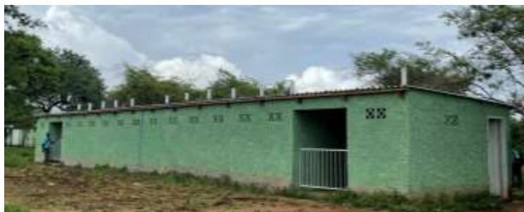
Student toilet block: for girls on left with 6 toilets and 1 shower, boys on right with 7 toilets plus urinals
